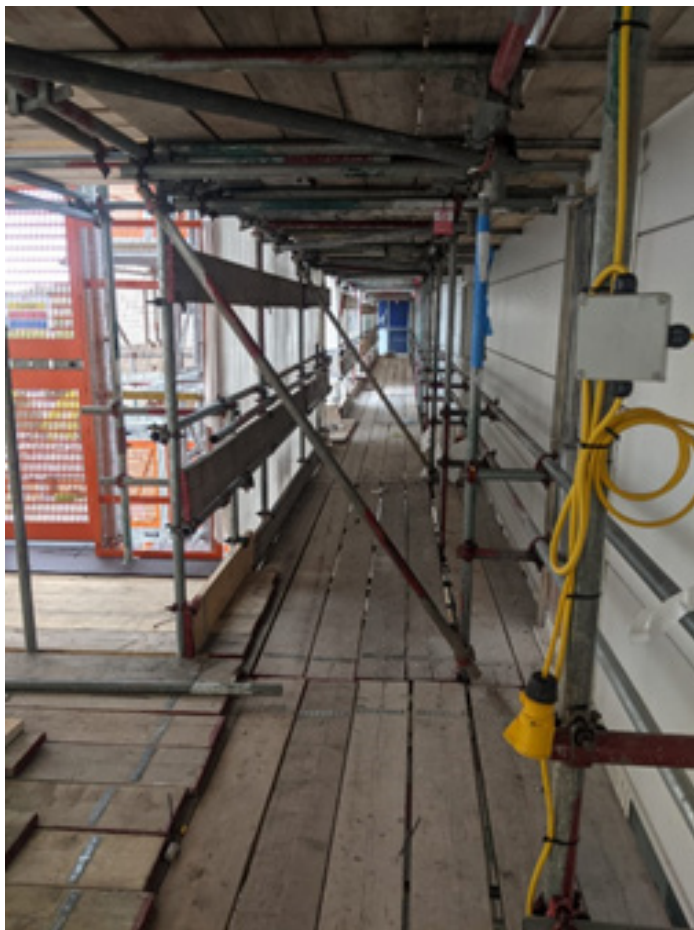
Light coloured building facade to be removed as a part of Shield's contracted works. External scaffold provided access for asbestos removal operatives.
