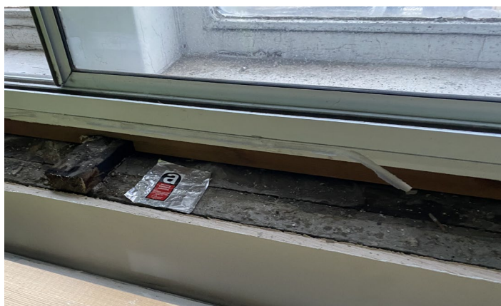
Example of AIB located to external windows.
