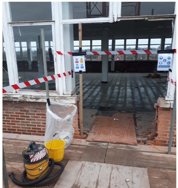
Access was cut in the exterior of building to provide access on to scaffold
