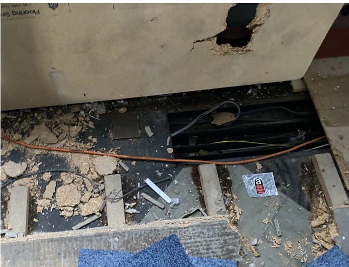
Example of AIB debris recorded to underside of existing floor.
