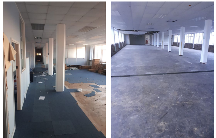
Pre and post images of soft strip works to floors of former office space.
