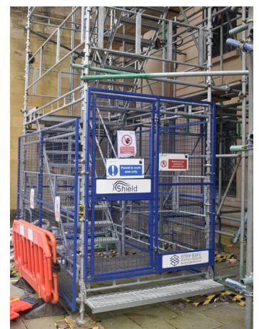
HAKI staircase with security gate
