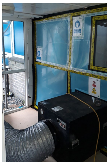
Right: Example of neagive pressure units to live enclosure
